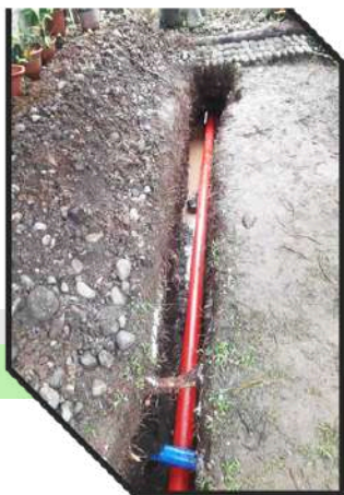
Drainage System at Executive House
